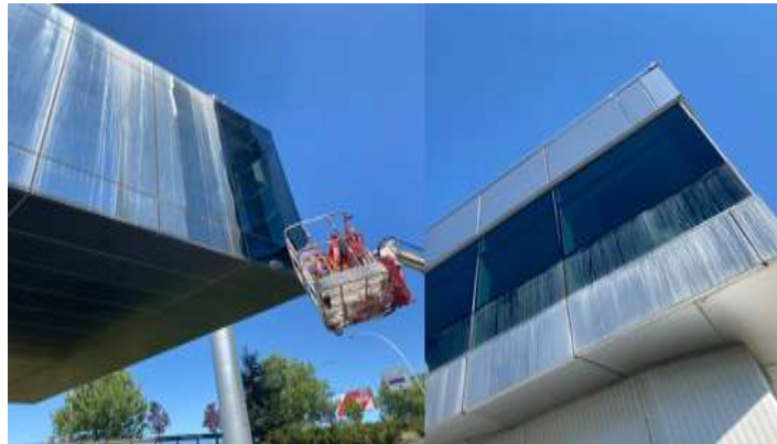
Figure 4: A building with dirty glass surfaces
